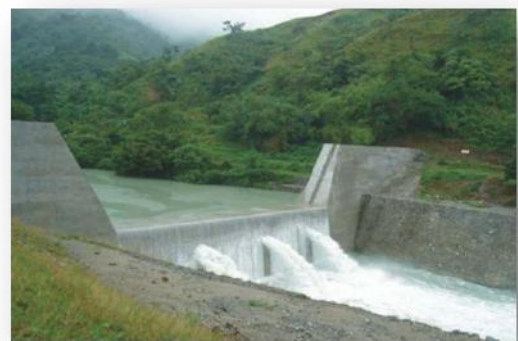
Gambar 3. Tipe Gravitasi Sabo dam sumber : Technical standards and guidelines for planning and design of sbao structures, JICA,Juni 2010
